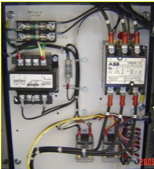
CONTROL PANEL BACKPLATE
